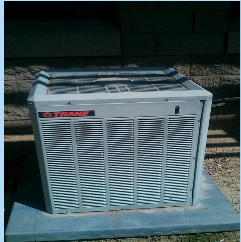
LCC – HVAC 200's/Gym/PAC
